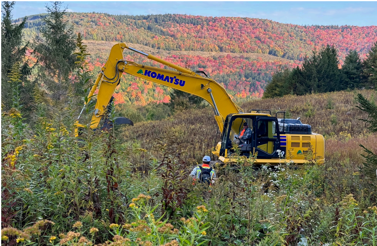
An excavator begins work on the decommissioning of sediment ponds at Cheat Mountain.
