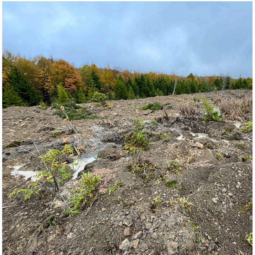
Post removal landscape in an area where one of the ponds was decommissioned.
