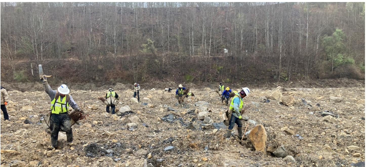
Clockwise from top left: A Komatsu 61PX bulldozer removes unwanted vegetation at the site. Freshly ripped and uncompacted soil is ready to be planted. Tree planting crew busy at work.
