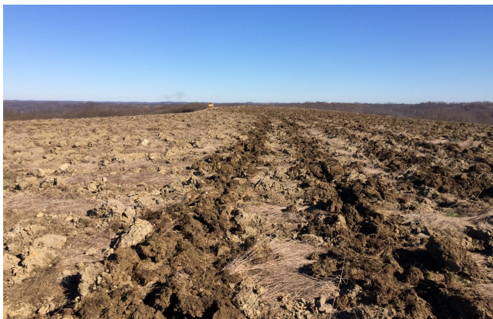
Figure 5. Rips in the soil after the first pass of the D9 with ripping shanks.
